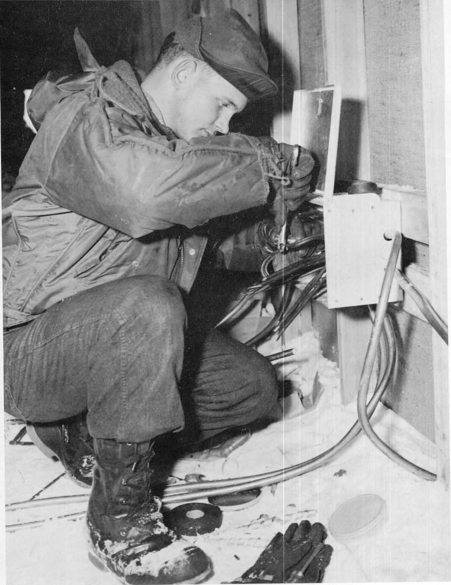
ELECTRICIAN PUSHES THROUGH LAST WIRING JOBS AT ELLSWORTH BEFORE THE SHIPS WEIGH ANCHOR.
