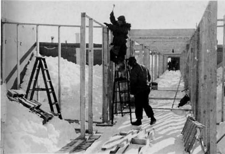
RACE against time finds MCB swinging hammers to raise interconnecting tunnels that will serve also as storage
