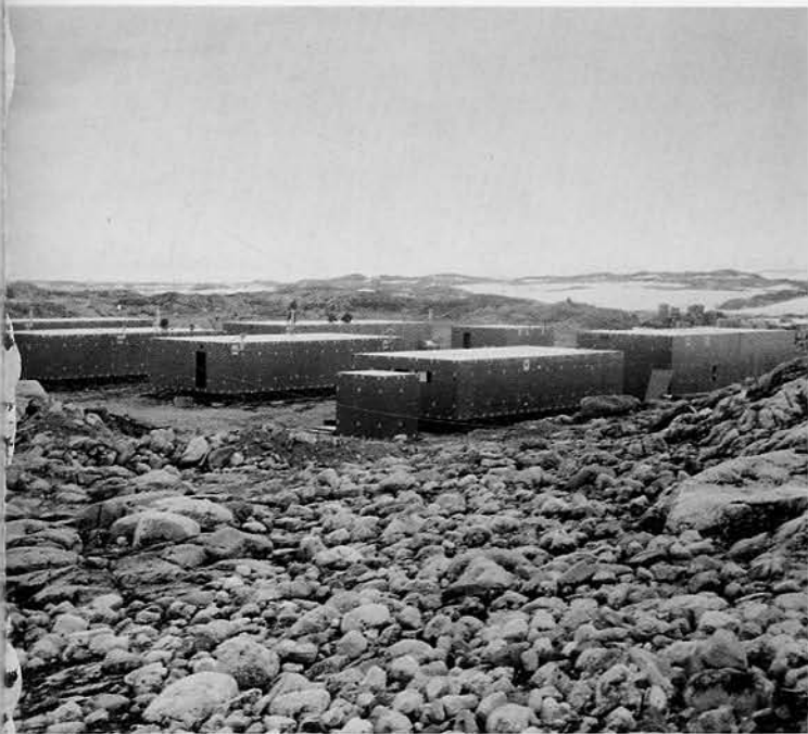
WILKES STATION in various stages of completion. Permanent structures (above) will house living facilities. Rawin dome (right) tops radar weather-balloon trackdown.
